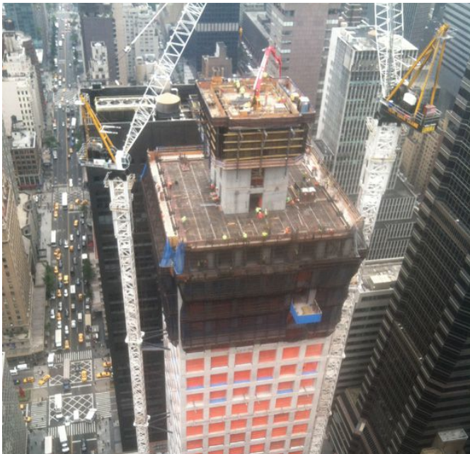
By the 20th floor, the project team lost the ability to use ground references. However, the Vertical Alignment System provided reliable control.
