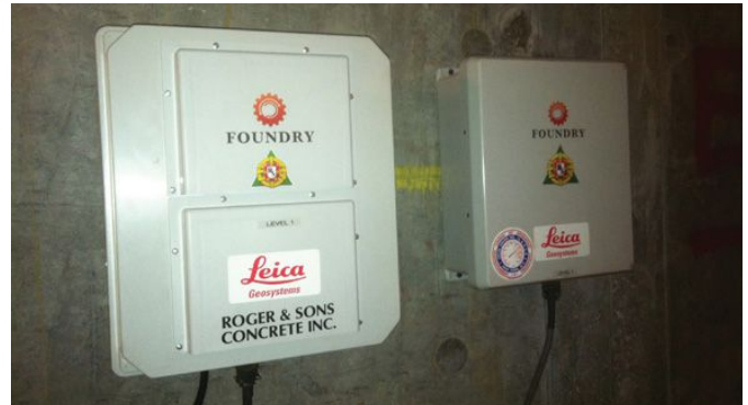
Leica Nivel200 Series dual-axis inclinometers, which can measure displacement to +/-0.2-inch of arc, are installed in the building's basement, and at regular intervals of about 10 to 12 floors to help predict the effects of the day-to-day construction and wind loads.
